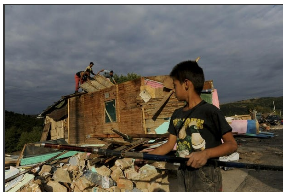
Members of the Roma community taking part in the demolition of the "Cesmin Lug" camp.
