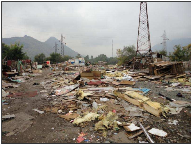
Camp Cesmin Lug demolished September 2010. Built by UNHCR and Norwegian Church Aid in December 1999 on toxic wasteland, it housed 38 families for 11 years.
